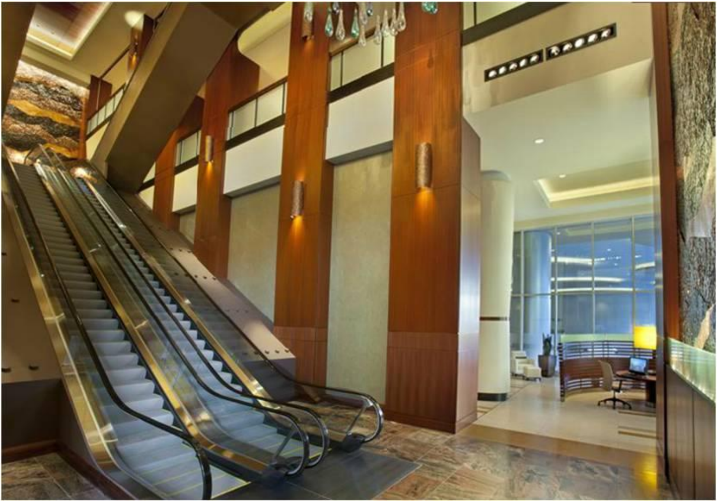
Hotel escalators at the ground floor
